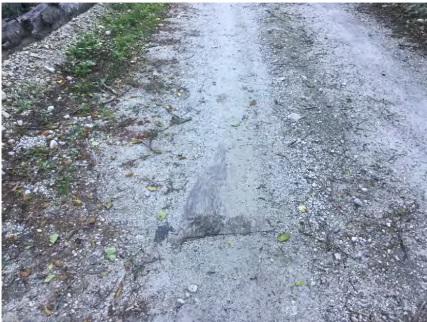
Right Abutment Top of Stringer Exposed
